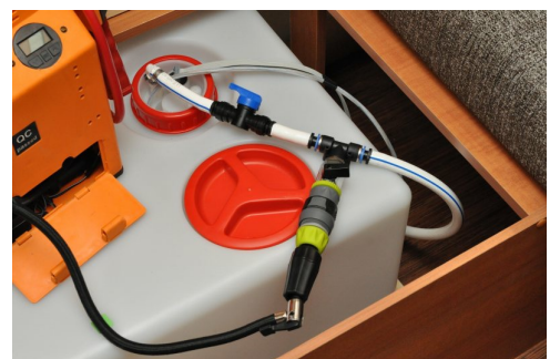
Keep Floeing drain down system
