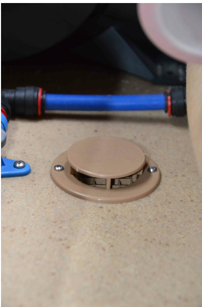
Opening up floor lockers encourages airflow through the van from drop out air vents
