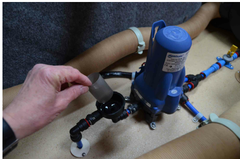
Clean grit filter while the system is empty
