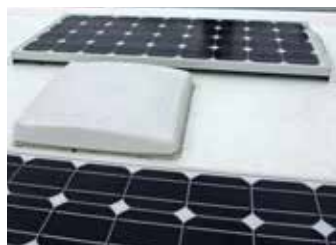
Solar panels are an excellent way of keeping a battery charged
