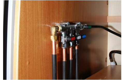
Gas valve manifold
